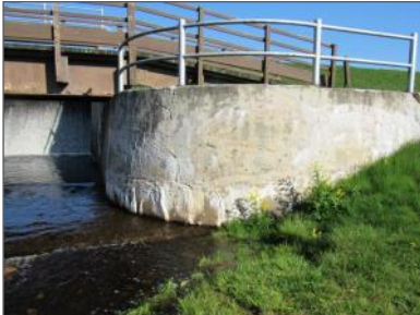
Crumbling dam at Tobyhanna State Park
